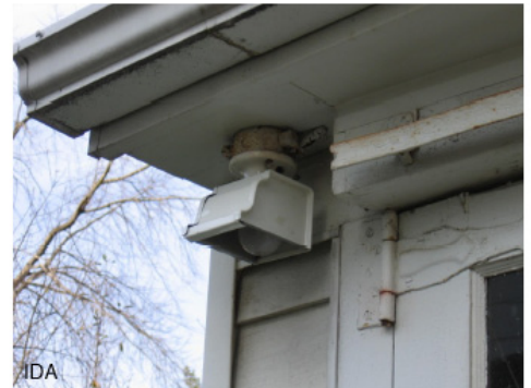
IDA Fixture shields can be made from household objects. This shield is made from a rain gutter.
